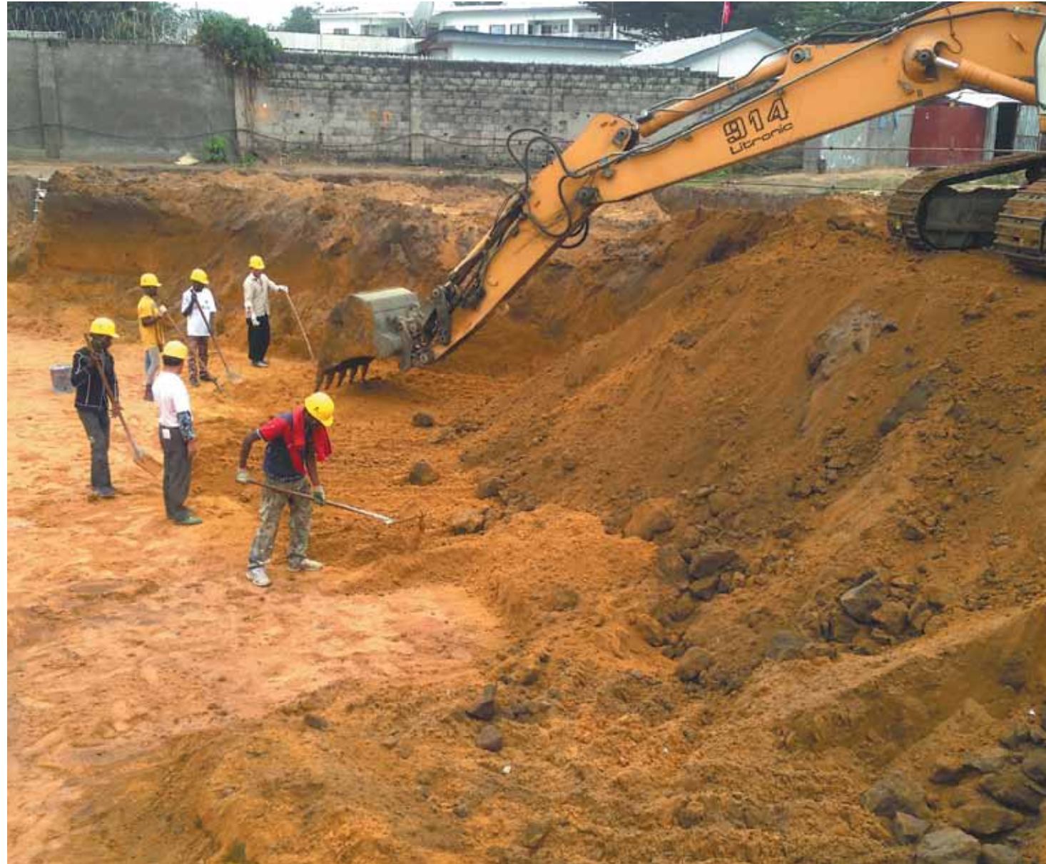
Employees of Beijing Uni-Construction Group Co Ltd (Congo) at a construction site in the Republic of Congo. ZHANG WEI / CHINA DAILY
